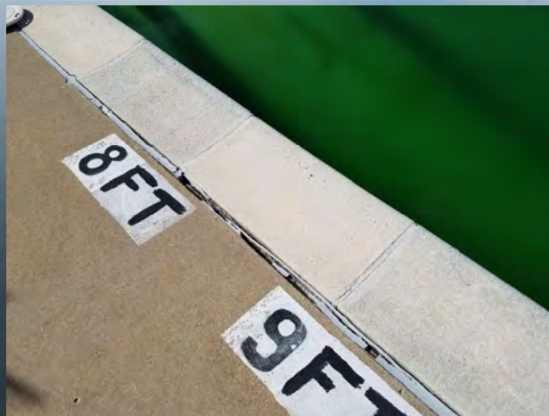
Broken sealant around coping
