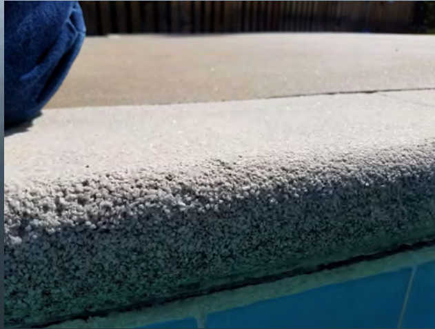
Cracked mortar bedding under coping
