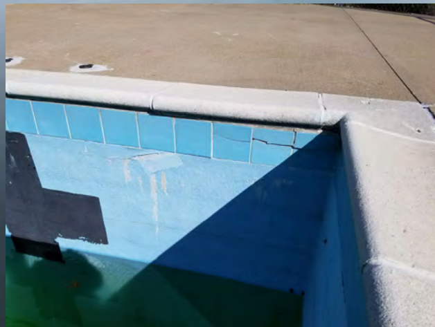
Cracked tile and peeling plaster
