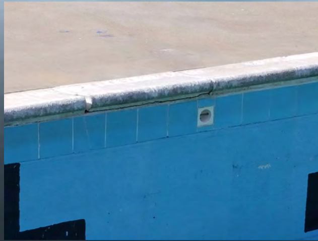
Cracked mortar bedding under coping
