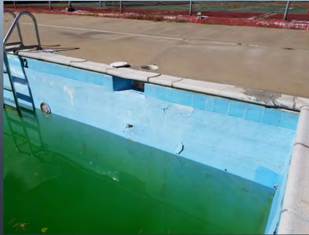
Peeling plaster lining
