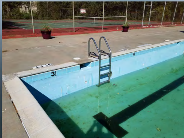
Peeling plaster lining
