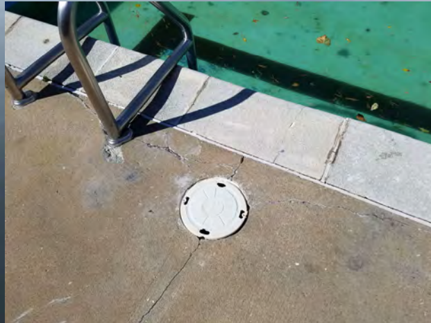
Skimmer and cracked coping
