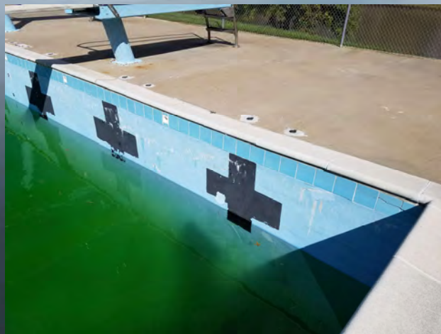
Cracked tile and peeling plaster
